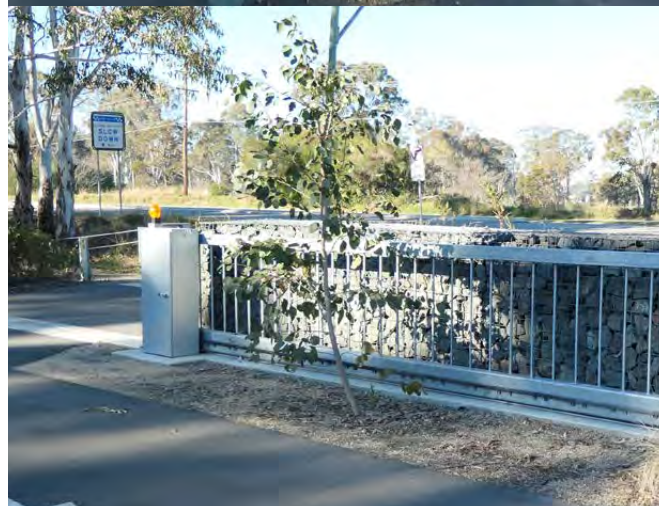
Figure 3.16 - Self sown trees that occur too close to path edges, signage, and other structures need to managed and sometimes removed before they create significant issues.
